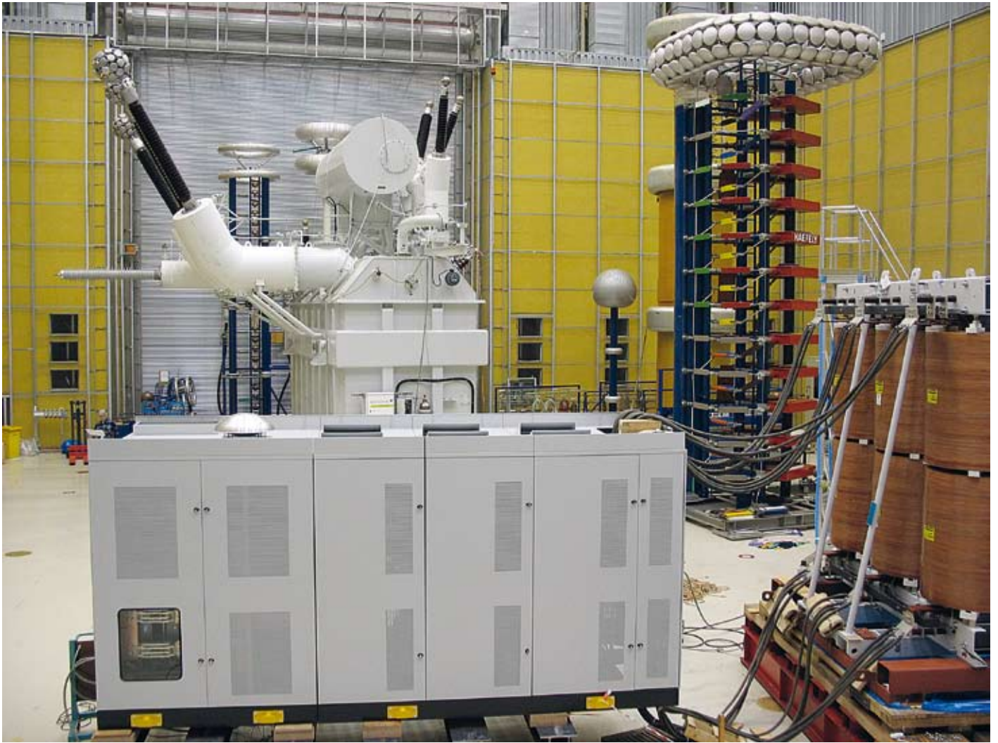
Test Field for non standard combined test of transformer and rectifier groups
